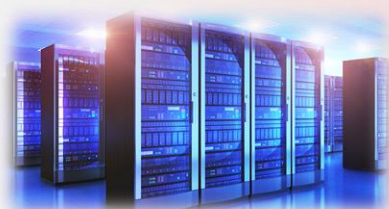
Data center & Logistic
